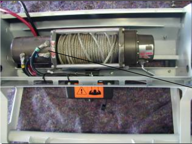
Photo above shows cable ties holding leads in place.
